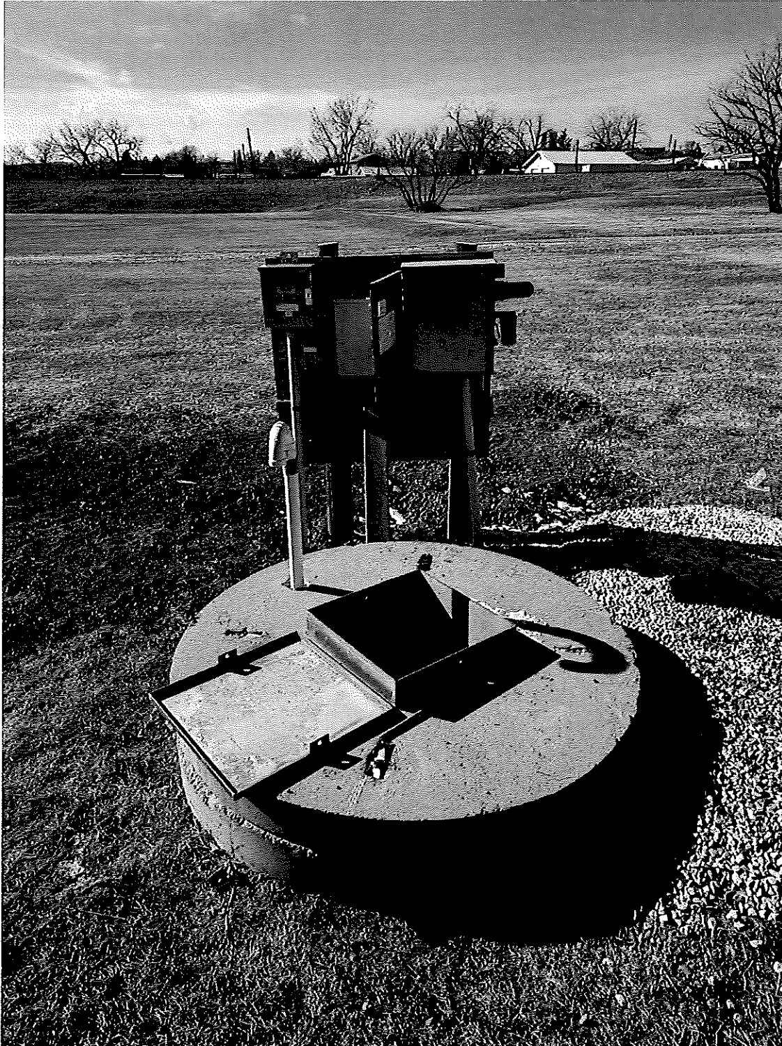
Figure 3. Ferguson Pump Station. Temporarily braced / non-code compliant repairs.
