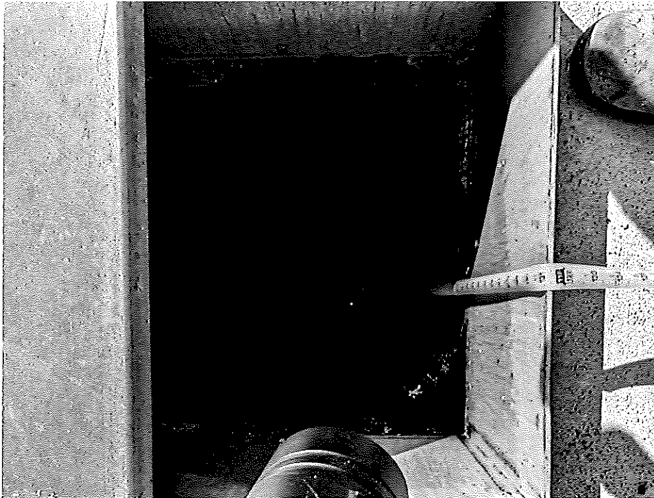
Figure 6. Wet well at 11 feet from rim (thus 7 feet full and 2 feet above inlet pipe).
