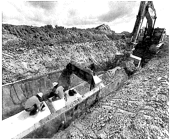
The construction timeline is largely dependent on the pace of state funding. At the current rate of funding, it could take 25 years or more to complete the pipeline.
