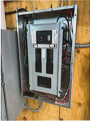
Breakers not marked.
