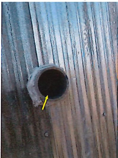
Mesh screen missing.
