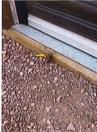
Rebar exposed at East side of building.
