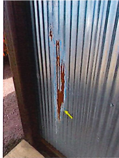
Small rusted area of siding noted at Northeast corner of building.
