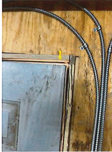
Air and light entering around door.
