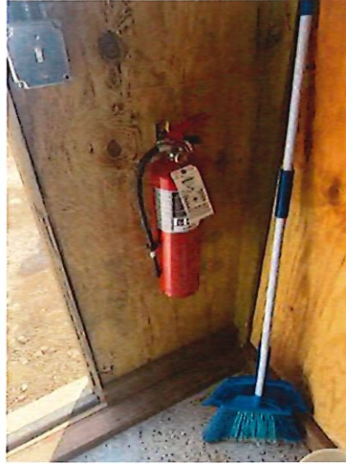
Fire extinguishers installed at both ends of building.
