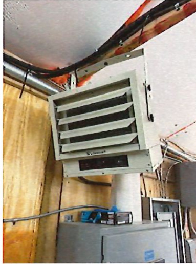
Electric heater functioning.
