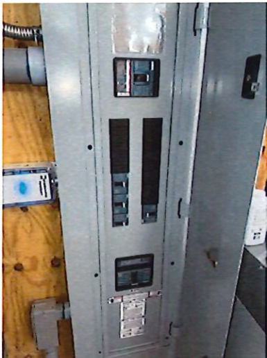
Breakers not marked.
