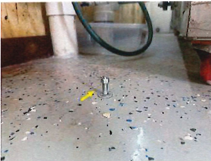
Bolt sticking out of floor.
