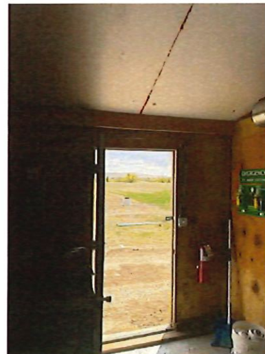
EXIT lights/sign missing.
