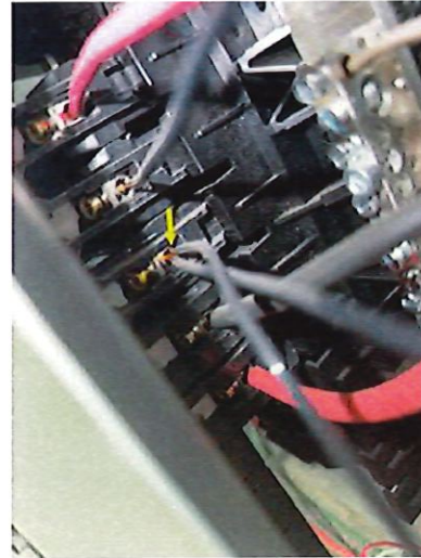
Double tapped breaker.
