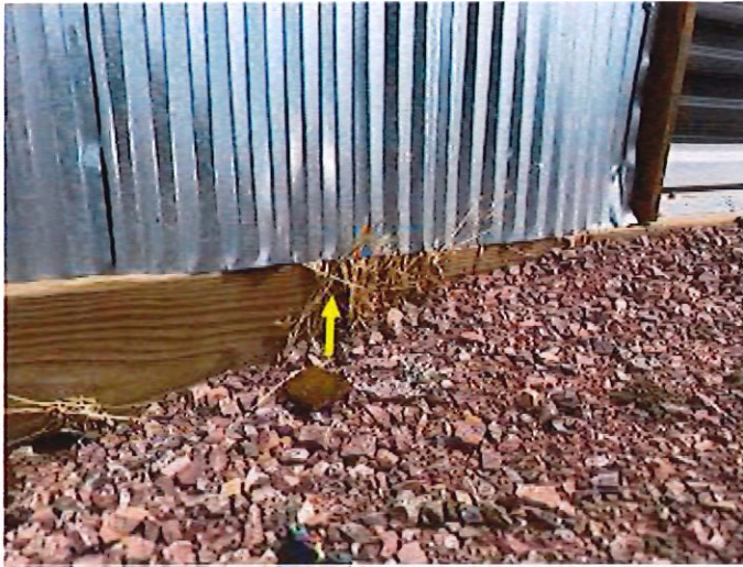
Weeds appear to be growing into siding.
