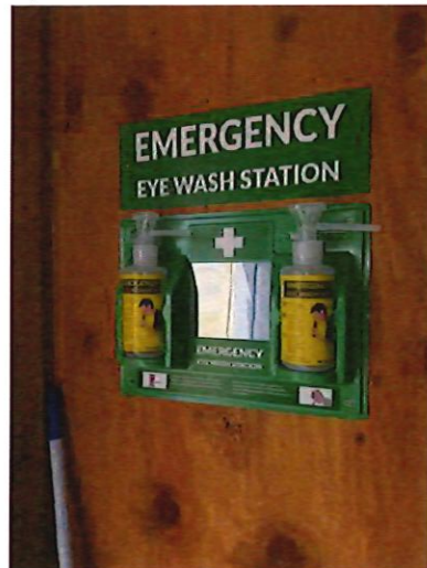
Emergency eye wash station installed.
