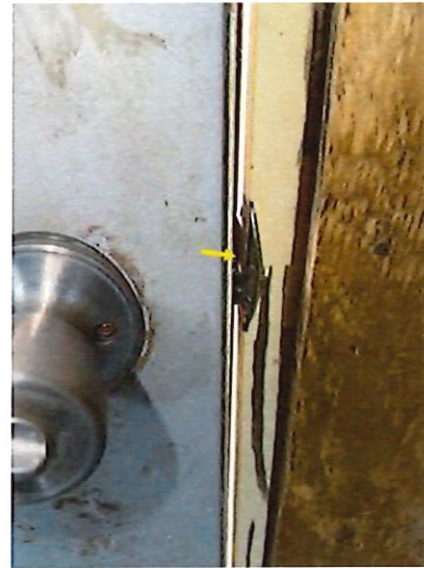
Door does not latch properly.
