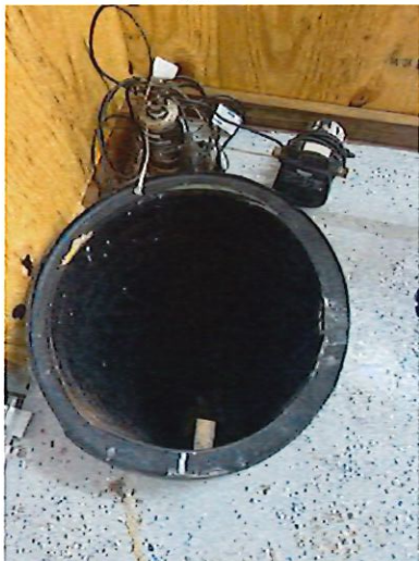
Sump pit cover missing.
