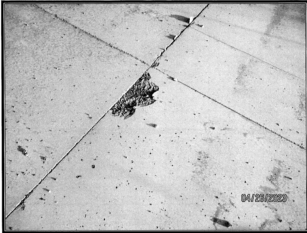
Outlet Apron Spall - Typical with Inlet Apron
