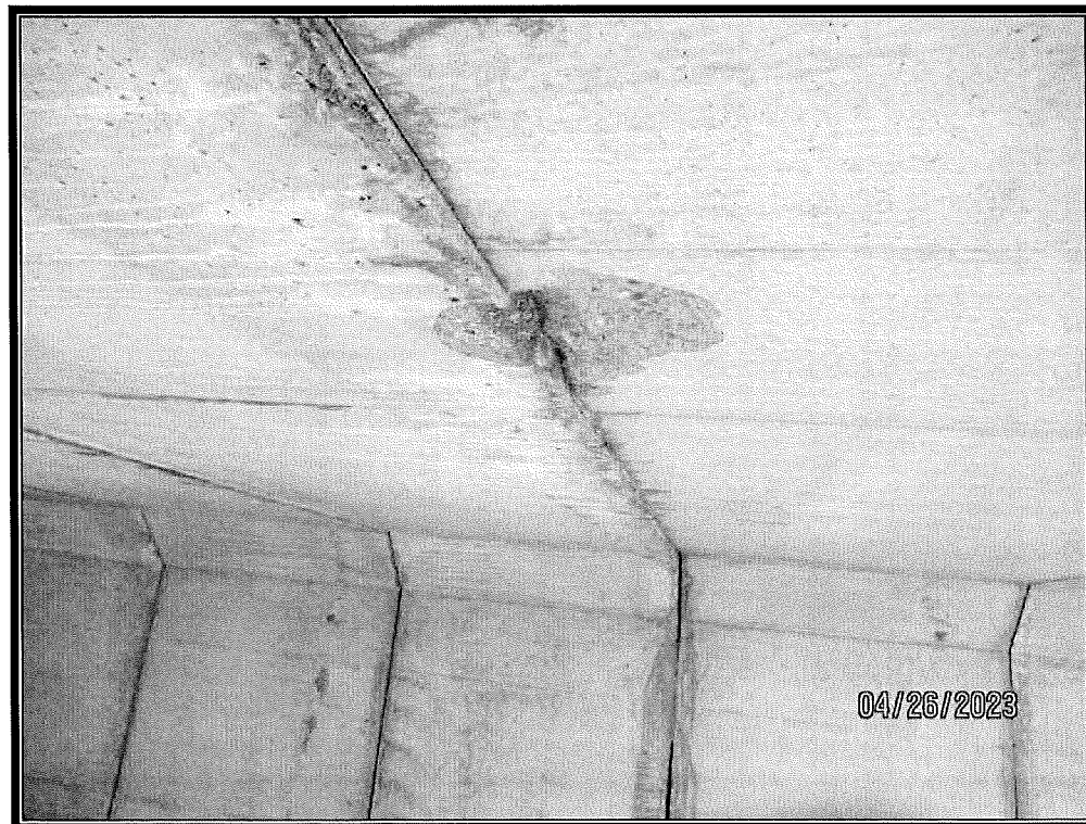
Top Slab Spalling - Typical
