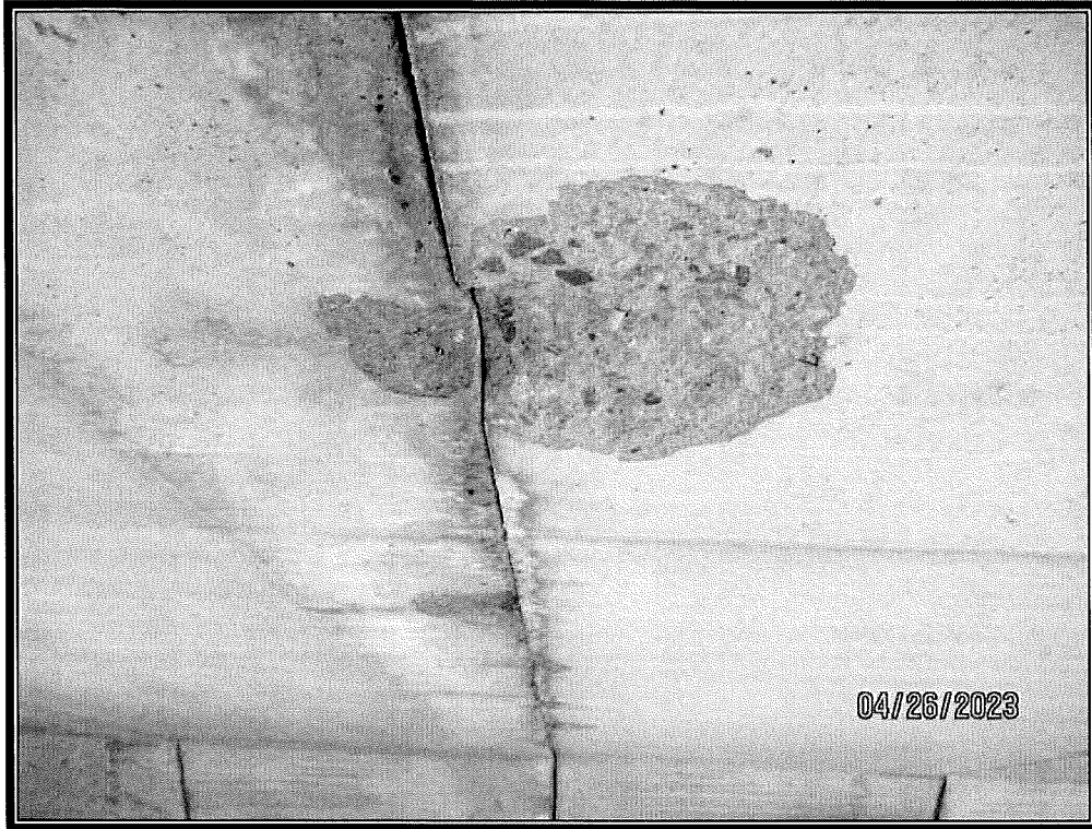
Top Slab Section 7 - Spalling with Exposed Rebar
