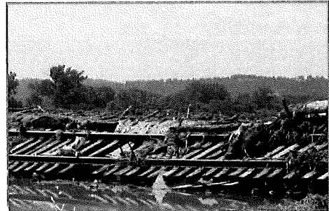
Image 4.7. Aftermath of Aug 2007 flood in Hermosa. DM&E railroad system damage. Image provided by Town of Hermosa.
