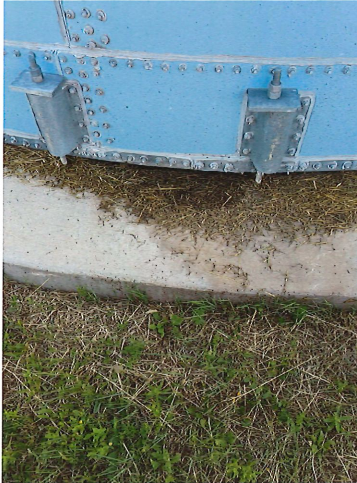
Figure 4. Photo taken July 3, 2024. Slow leak in 314,000 gallon tank that requires repair.
