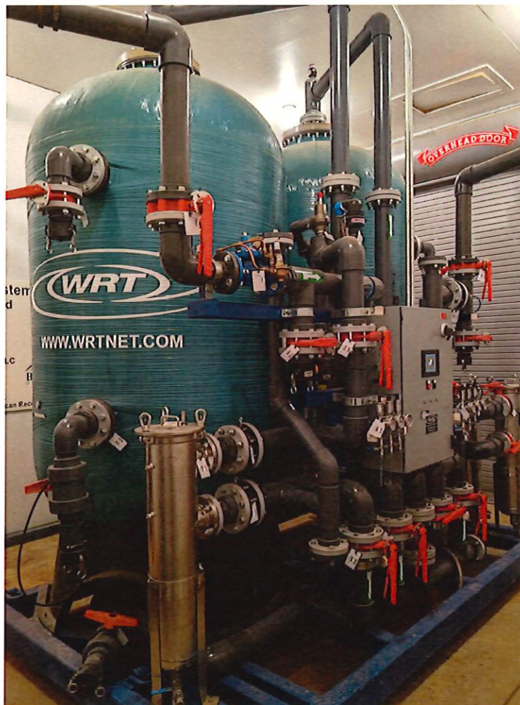
Figure 2. Water Treatment Plant (Photo is of the system operating in New Underwood, SD).
