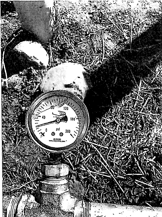
Photo 1: Static pressure at existing fire hydrant.
