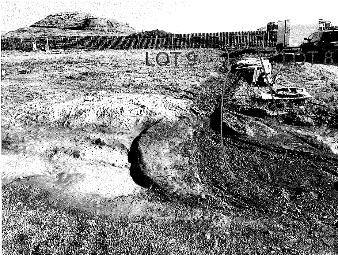
Photo 1: Contributing flow drainage path into Hermosa Hills from the property to the north, illustrating significant sedimentation buildup causing re-channeling of the existing drainage ditch. View North from Marie Street, along the property line of Residential Lots 8 & 9.
