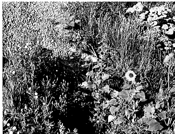
Photo 3: Marie Street 18" CMP Inlet partially crushed.
