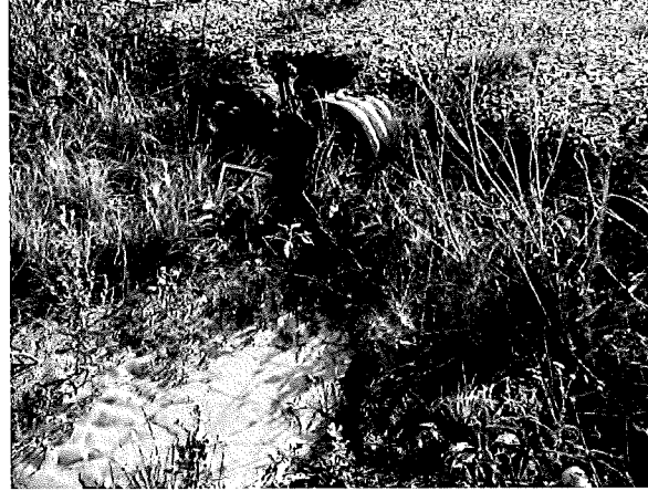
Photo 5: Obnoxious weeds at inlet, view NE
