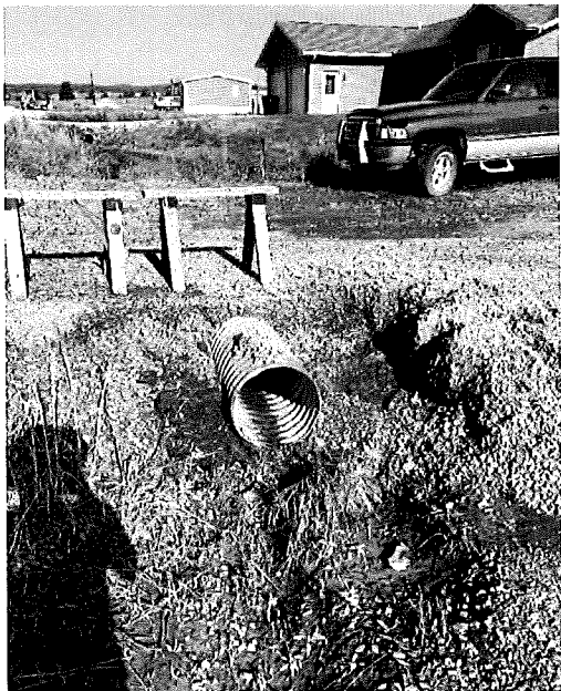
Photo 7: Driveway degradation and washout at culvert outlet, view west
