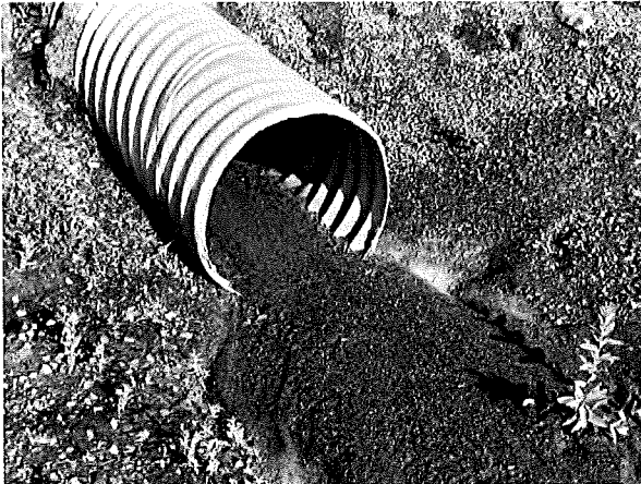
Photo 4: Culvert with sedimentation, view NW
